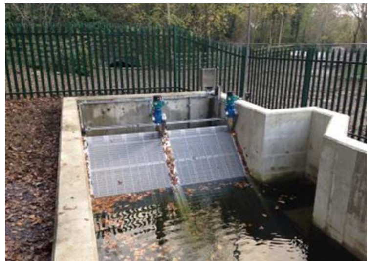
The GoFlo travelling screen at the hydro intake
