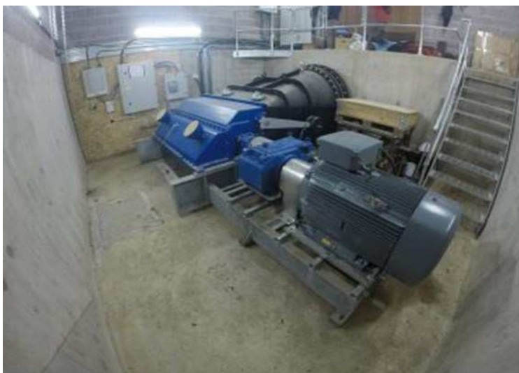
90kW Crossflow turbine
